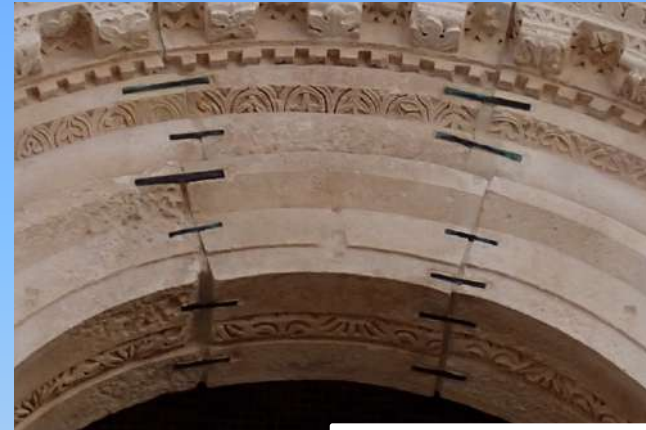
Current damage of the real structure
